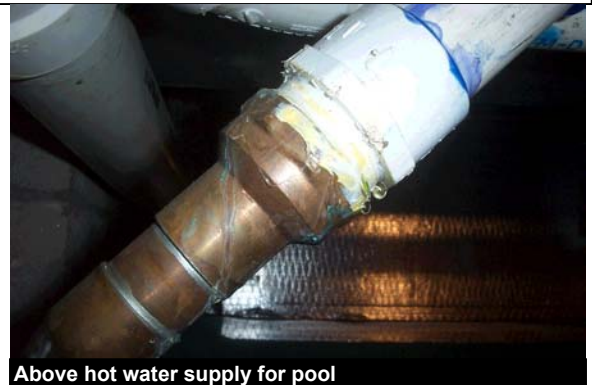
Above hot water supply for pool
