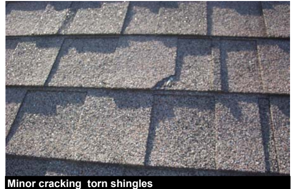
Minor cracking torn shingles
